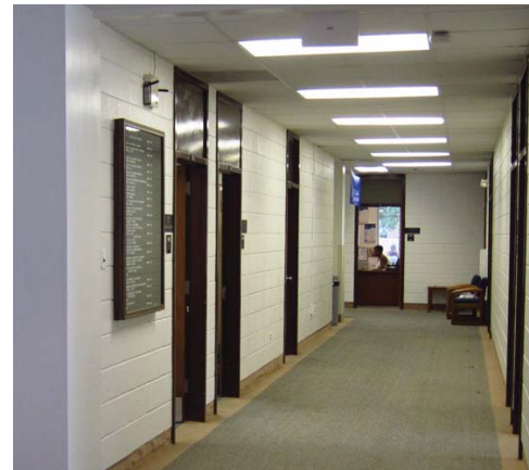
Typical corridor - note attempt to make corridor more inviting by furniture placement. This occurs in several of Kent Hall's corridors
