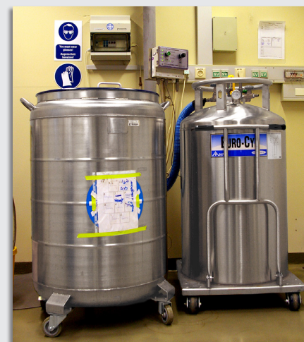
Liquid nitrogen tank
